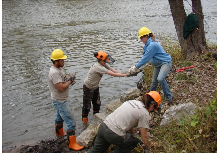
Portage construction involving hand-placed stones at a launch downstream of a dam.
